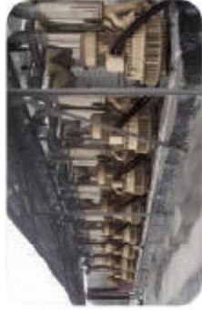
Welding fume extraction
